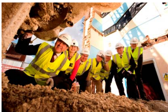
PHOTO 2 below: August 2010 -Work on the foundations begins Alabaré Ambassador and Lord Lt of Wiltshire John Bush joins representatives from the partner agencies on site to see the foundation works take shape.
